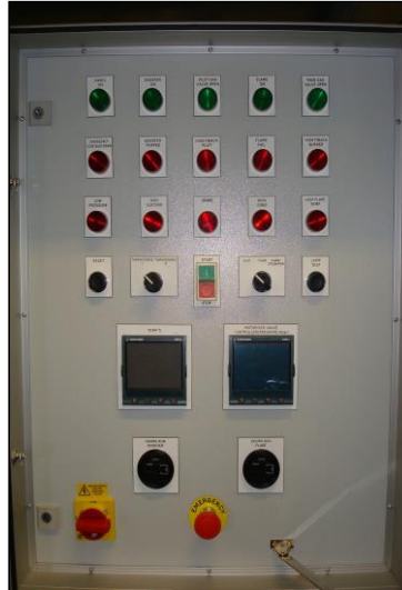
Wide range of control systems
