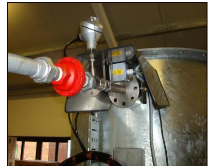
Fireblaster landfill gas Pilot
